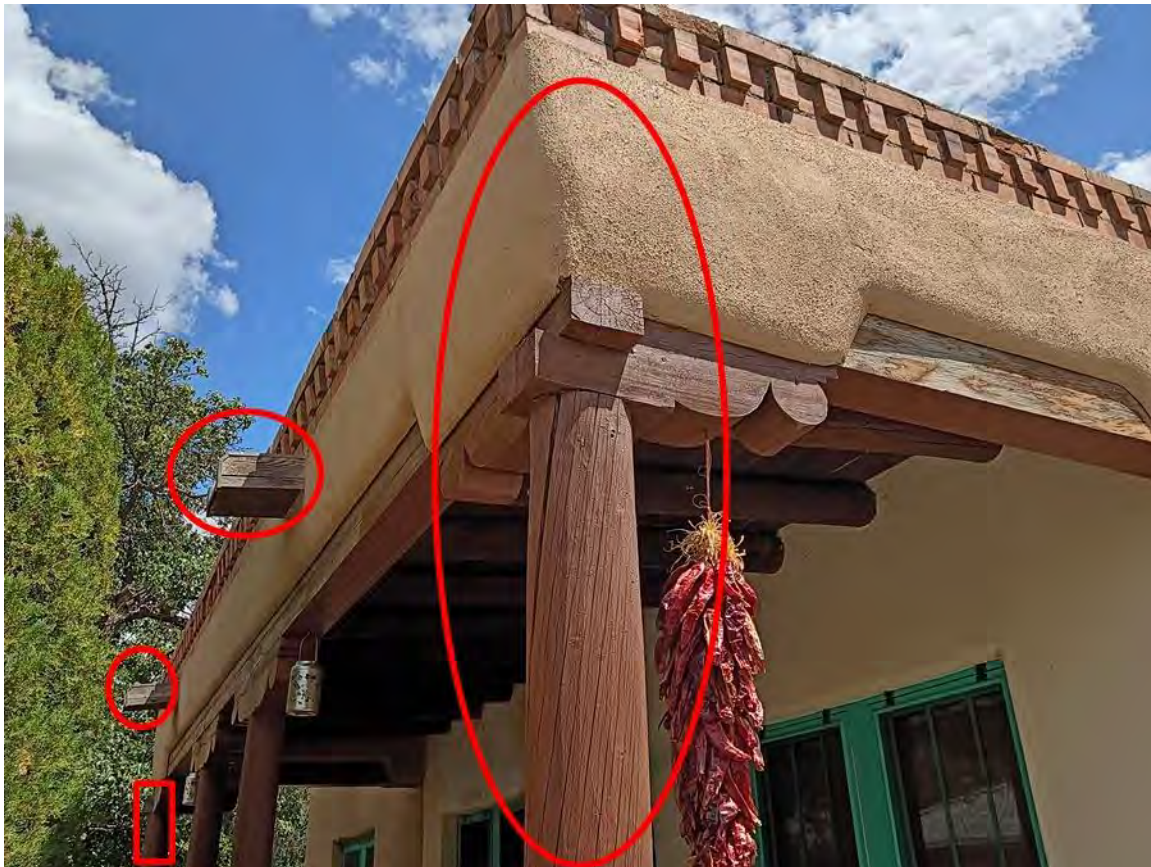
Photo 5: Elements that have been altered across the portal. Camera facing up.
